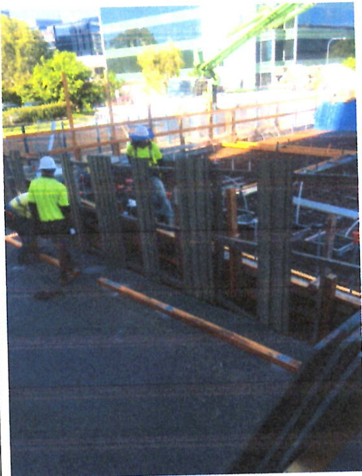
Evelyn St bin access driveway, dismantling common wall to allow access to build new wall. Image taken 31-01-17
